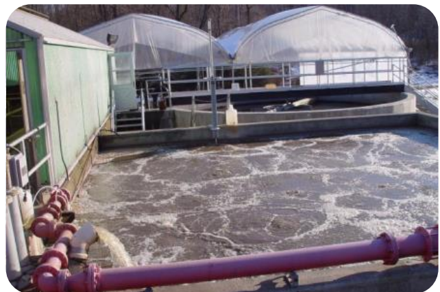
Philmont's waste water plant
